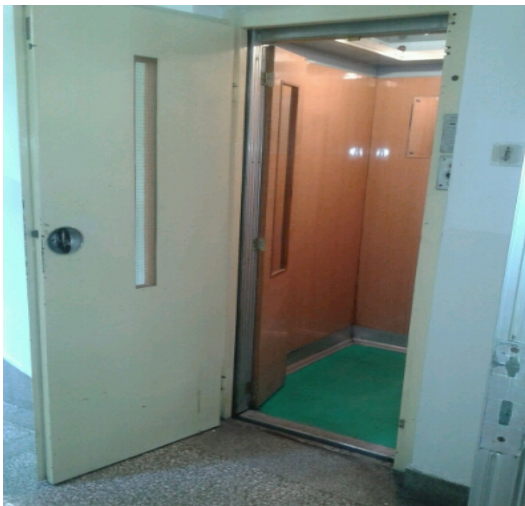
Figure 2.3. Elevator in the main building
