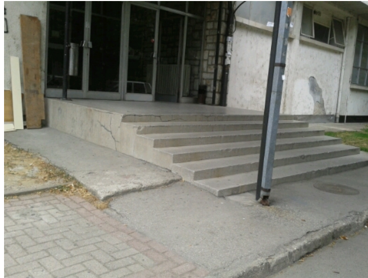
Figure 2.2. Entrance to the annex building with no ramps
